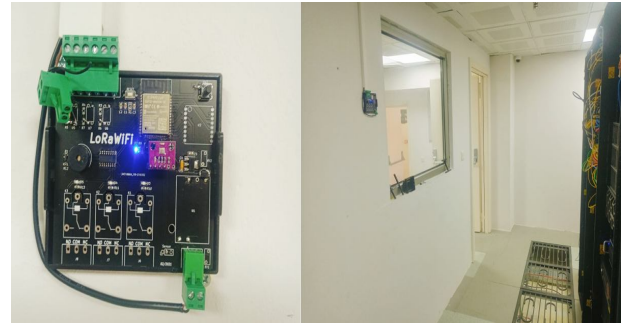
Fig. 4 View of the developed circuit from the server room
